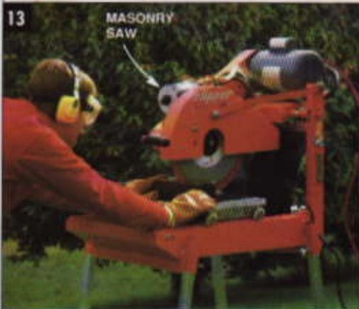
CUT PAVERS on masonry saw. Saw has a built-in sliding carriage for moving pavers past the blade. Recirculating water keeps blade cool and lubricated.
