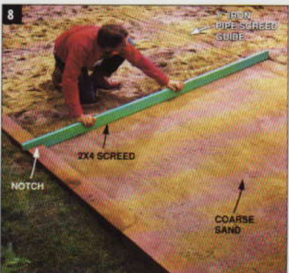
8 SPREAD AND LEVEL a 1-in. bed of sand over compacted subbase. Pipes provide a guide for dragging the 2x4 screed board across.
