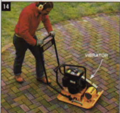
TAMP THE PATIO with a flat-plate vibrator after all the pavers are installed. Tamp entire outside edge first, then circle in.
