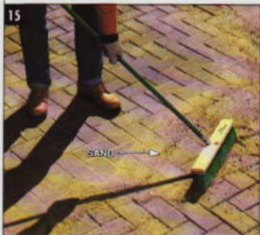
SWEEP COARSE, DRY SAND between cracks of pavers to lock them together and fill voids. Repeat with more dry sand in a few days.
