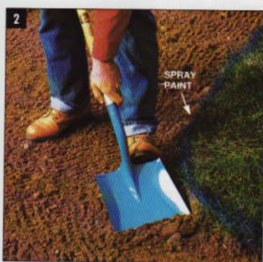
2 REMOVE SOD in an area extending 8 in. beyond the boundaries of the patio. SPRAY PAINT indicates the excavation line.
